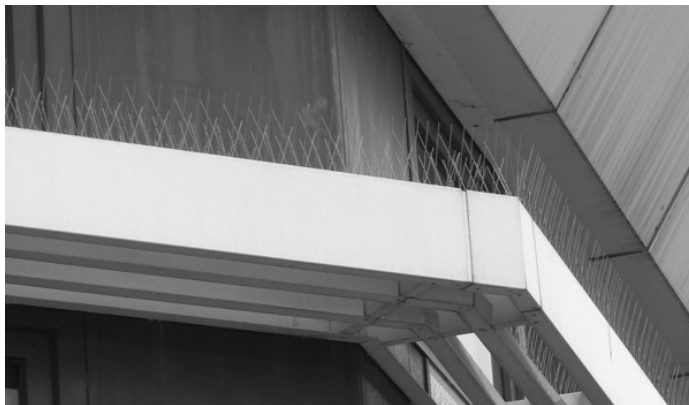
Photo 1. Protecting nets on cornices of the SGGW building
